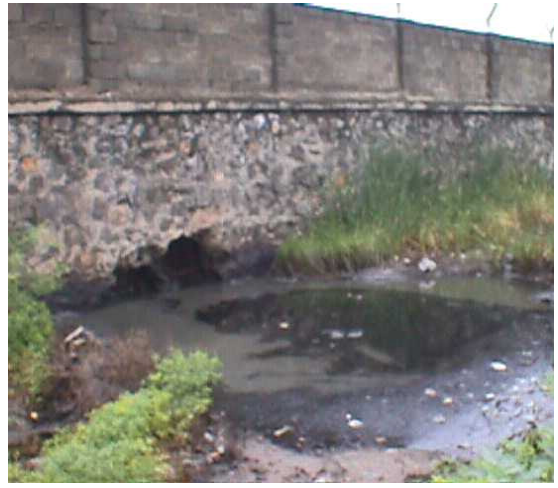
SPREAD OF ASHOK LEYLAND EFFLUENT ACROSS COMPOUND WALL INTO BUCS BANKS
