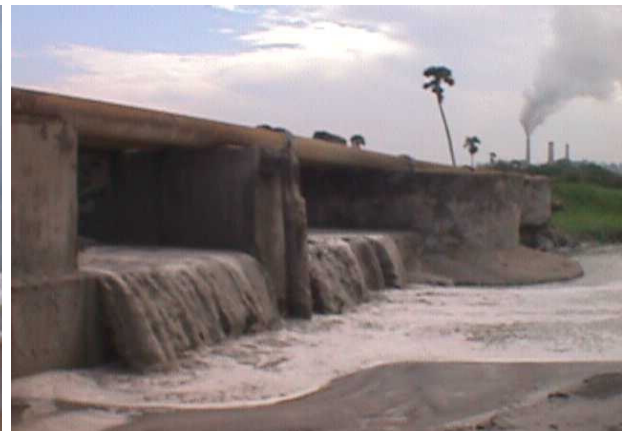
ETPS OUTFALL DISCHARGING COOLANT WATERS THE PIPELINE ABOVE THE OUTFALL CONVEYS FLYASH SLURRY FOR DISPOSAL FURTHER OFFSHORE
