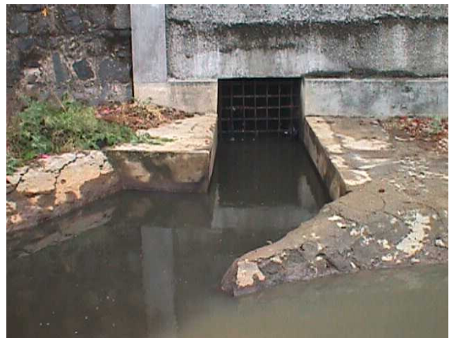
ONE OF THE EFFLUENT DISCHARGES IN THE AMULLAVOYAL CANAL
