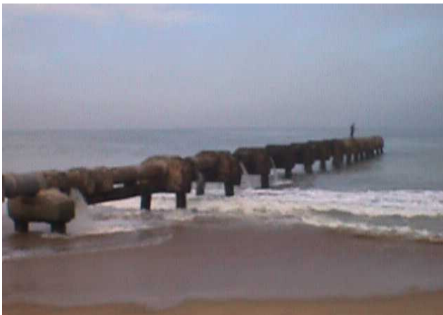
FRACTURED EID PARRY OUTFALL
