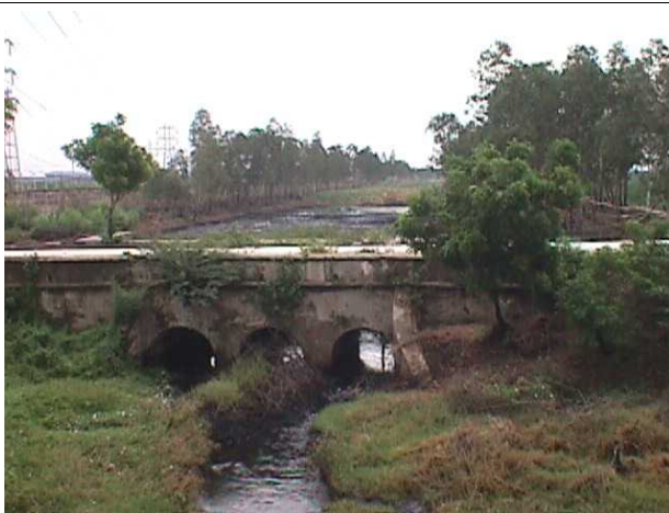
MRL OIL EFFLUENT OUTFLOW FROM FACTORY INTO BUCS
