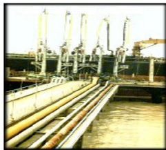
Pipeline for liquid cargo transfers
